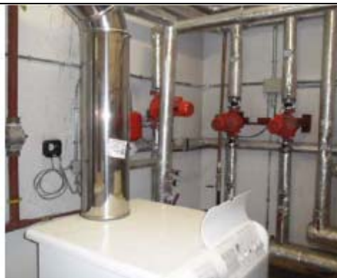
Sala calderas gas natural
