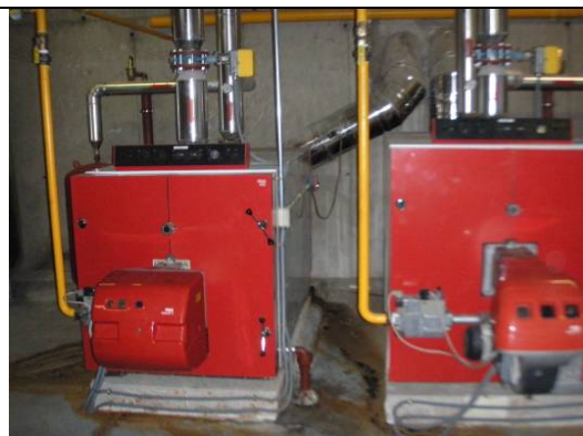
Calderas Gas natural
